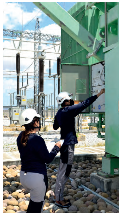
Operators at one of the plants in Mexico.
